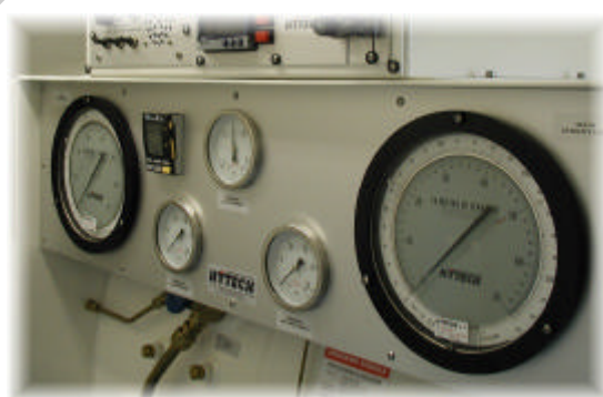
DDC control panel with gauges
