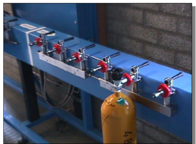
Filling station with stainless steel HP manifolds
