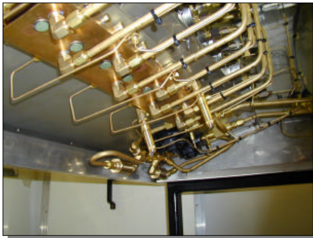
Air distribution manifold for Life Support Panel.
